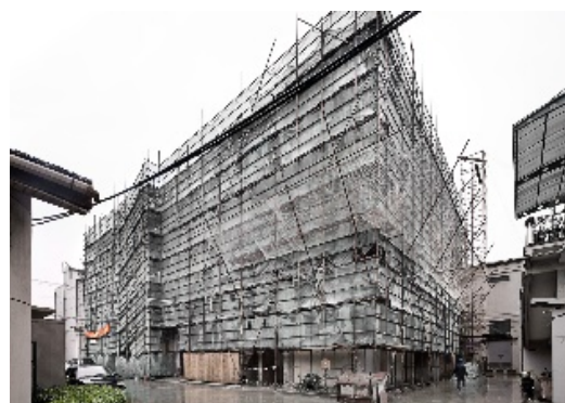
Figure 4.27: Construction View of the Main Building during Transformation of the Glass-Making Factory into SHMOG (Url 4.37)
