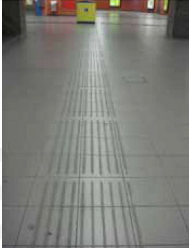
4.1.16. Embedded Directional Metal Bars (Brussels, Belgium)
