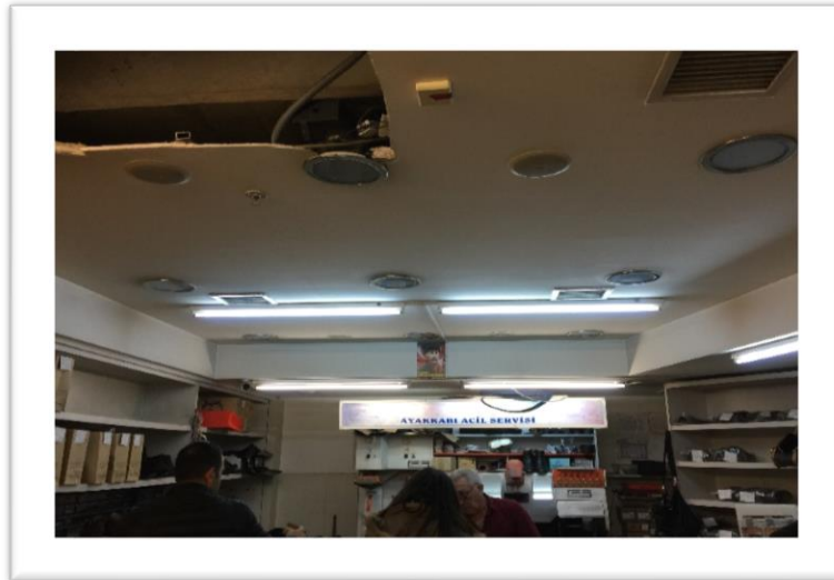
Figure 3.7: The General Lighting of SR 4 (Photograph taken by the author)
