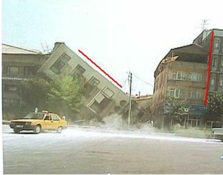
Figure 2.5. A building in Adapazarı that fall over in the 1999 earthquake due to soft ground it is constructed on.
