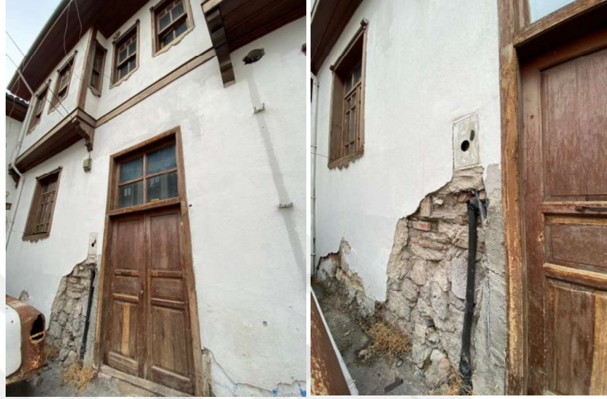
Figure 39. Hamamönü Region, Ankara House Stone Material, Simple Console Projection, Windows, Eaves, Entrance Door and Top Window (Author's Archive, 2021)
