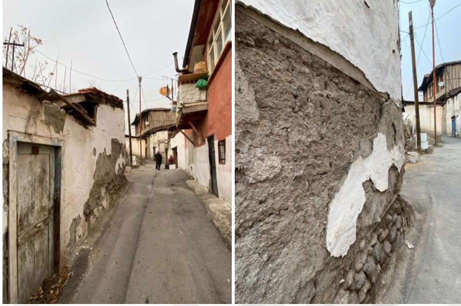
Figure 41. Hamamönü Region, Ankara House In Ruins Stone Material, Courtyard Door, Street Buildings (Author's Archive, 2021)
