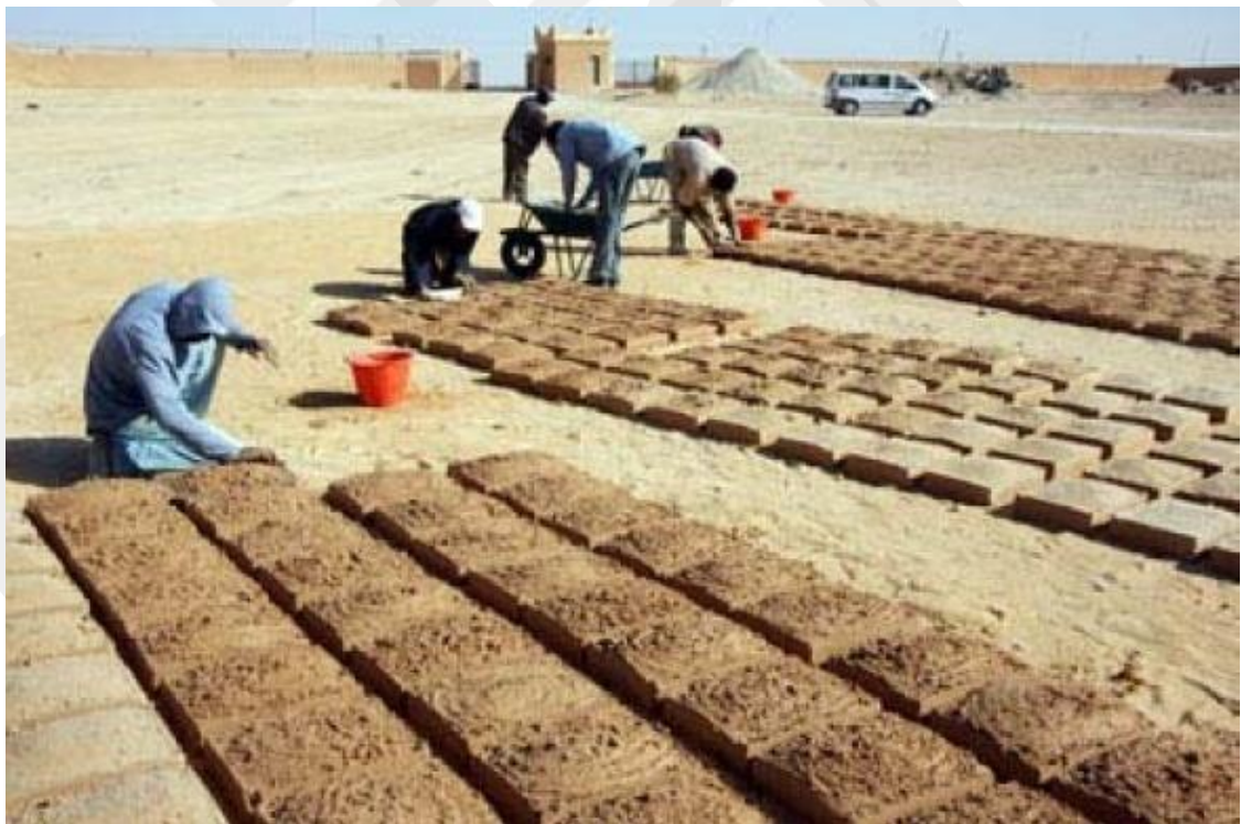
Figure 3.30: Adobe bricks production as part of the restoration works (Auroville Earth Institute, n.d.)
