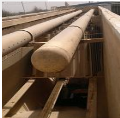
Figure 1.2 Inside sedimentation basin for compact unit
